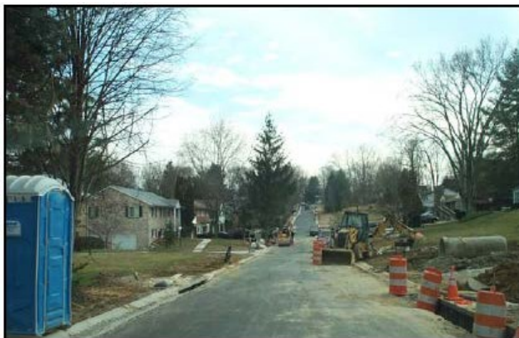
Figure 3-5: Roadway Repairs and Maintenance Generating Significant Amounts of Sediment
