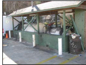
Covered/Contained Fuel Tanks
